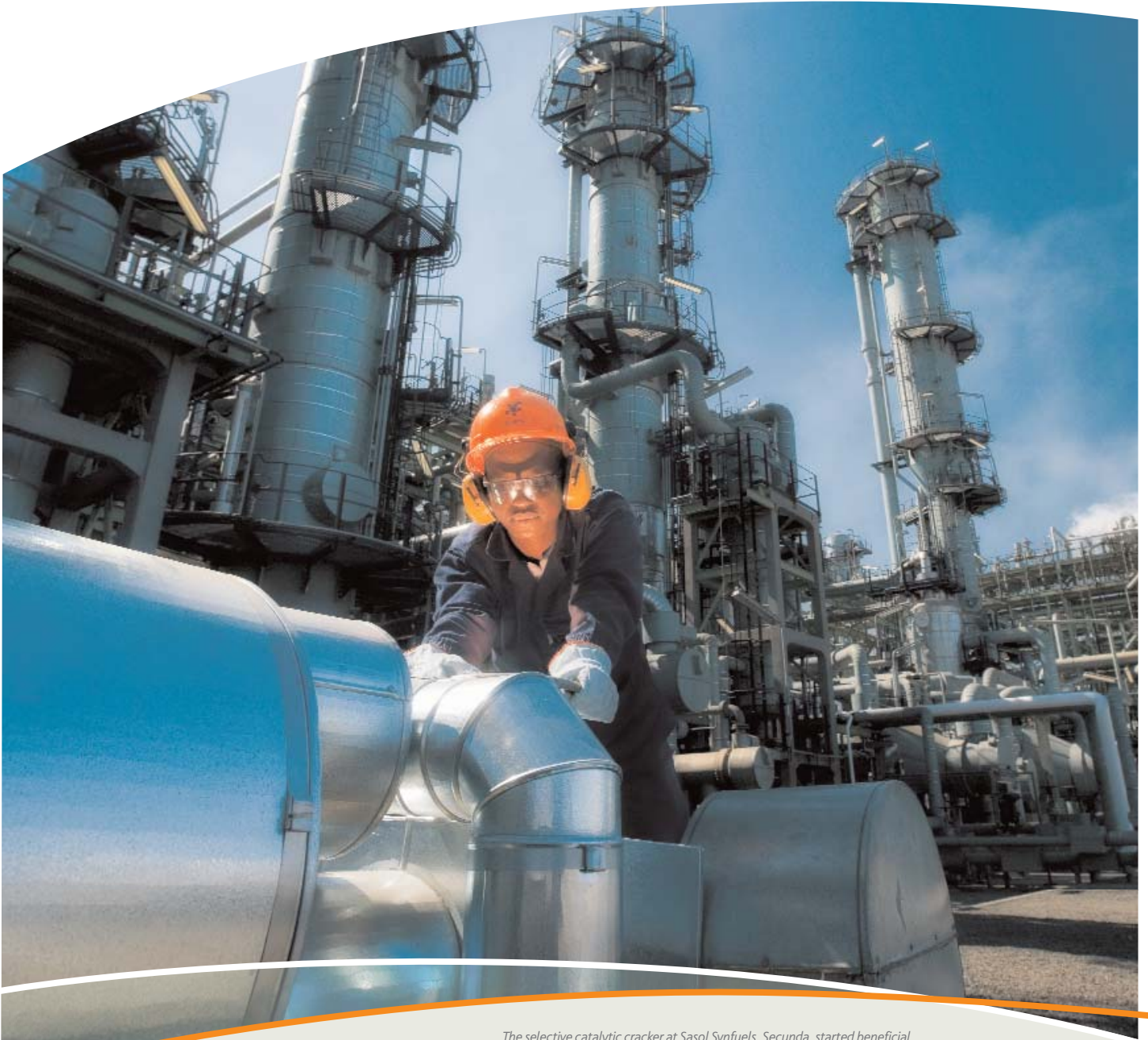
The selective catalytic cracker at Sasol Synfuels, Secunda, started beneficial operation in January 2008.
