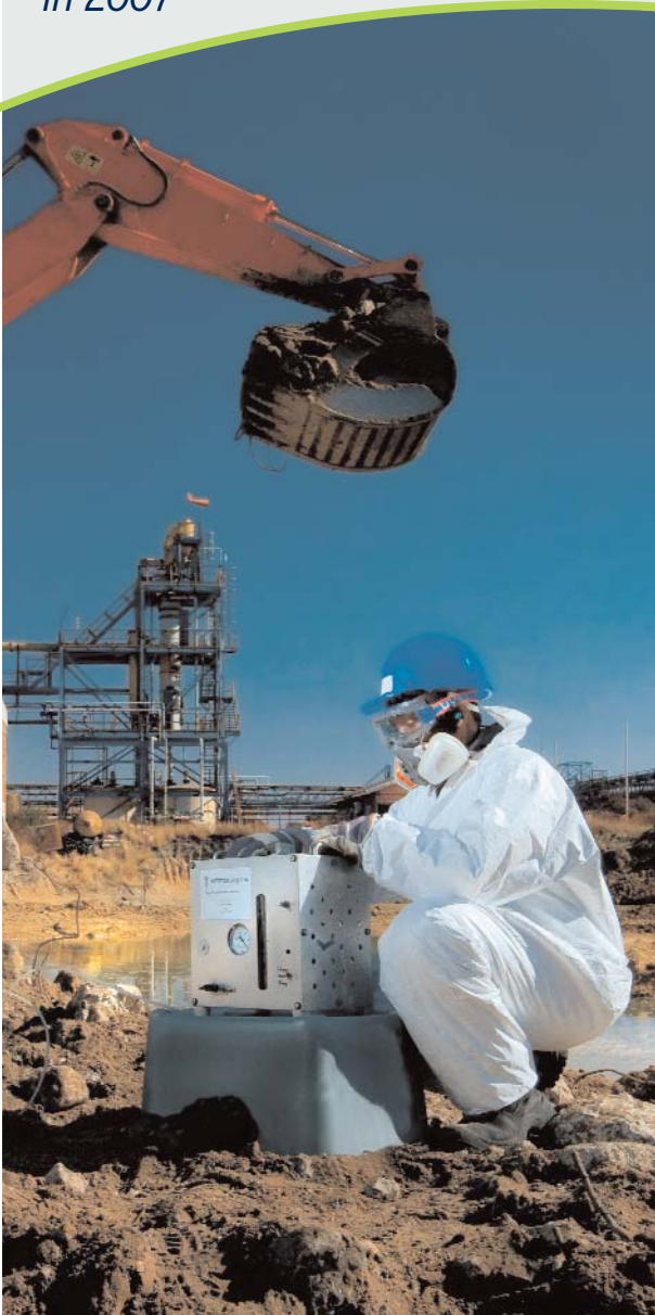
We undertake regular monitoring of contaminated land.
