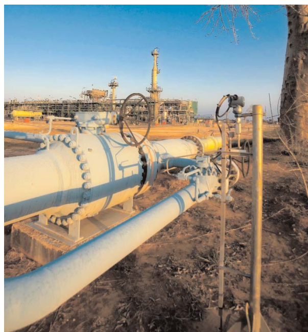
Central processing facility, Temane, Mozambique.
