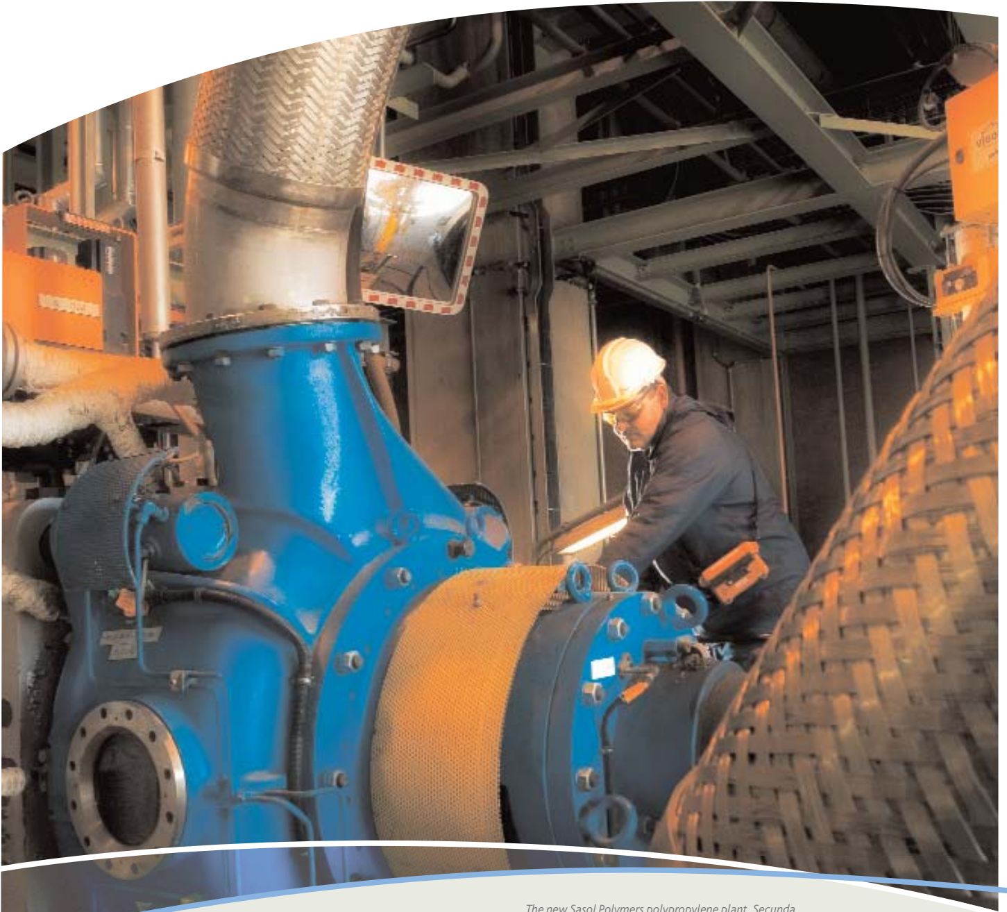
The new Sasol Polymers polypropylene plant, Secunda, started beneficial operation during the year.
