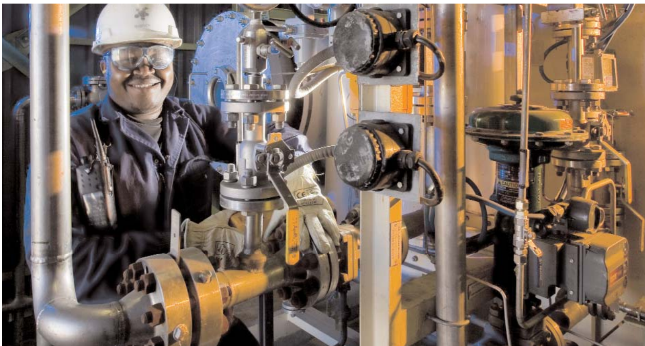
Pule Letuba, process controller at the Secunda water recycling project, checks the ozone generator unit.
