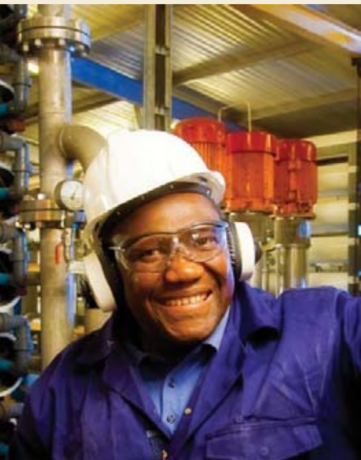
Aarom Mahlangu at the reverse osmosis unit for water purification of Infrachem at the Midland site.
