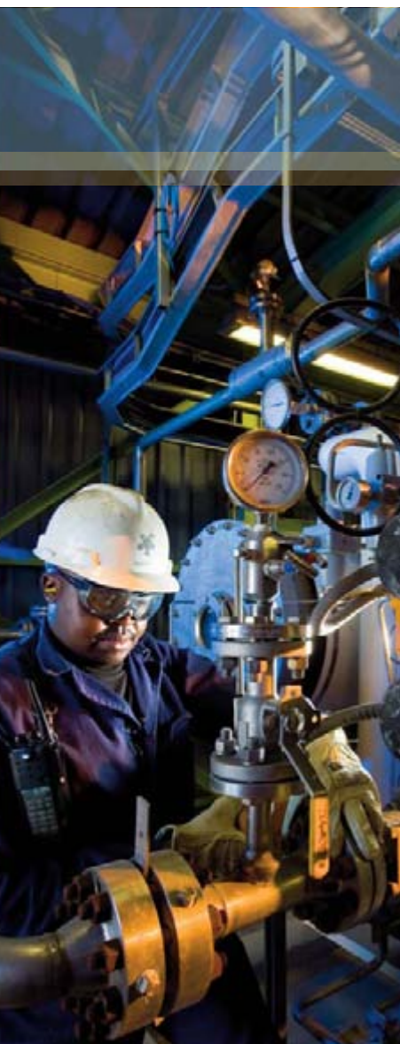
Pule Letuba , process controller at the Secunda water recycling project, checks an ozone generator unit
