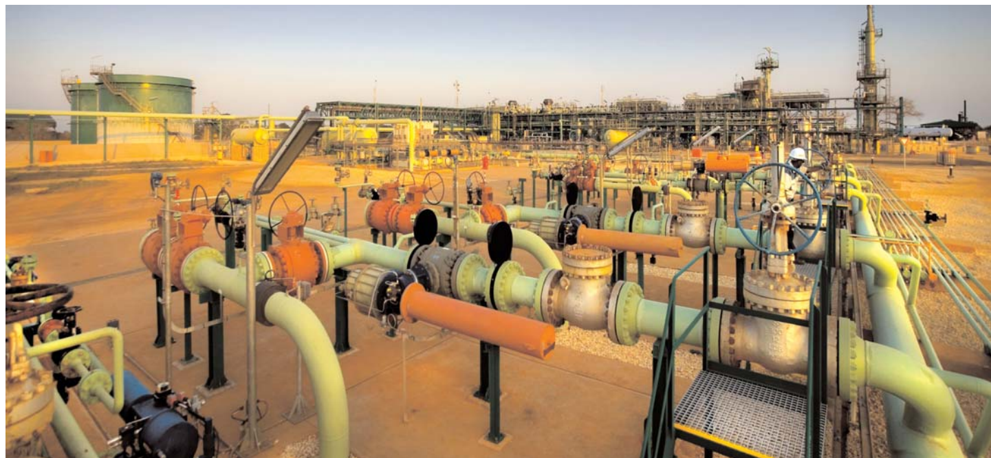
The central processing facility at Temane in Mozambique where capital expenditure is expected to allow for increased gas volumes.
