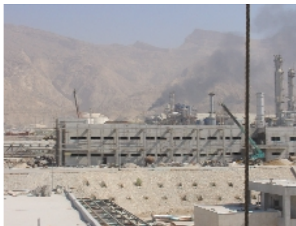
The Sasol Arya monomer and polymer production facilities at Bandar Assaluyeh in Iran will be completed in 2006
