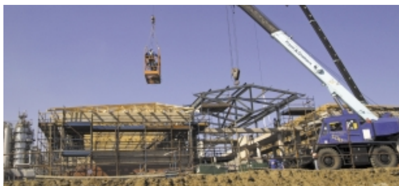
A view of work in progress for the construction of the new selective catalytic cracker at Secunda
