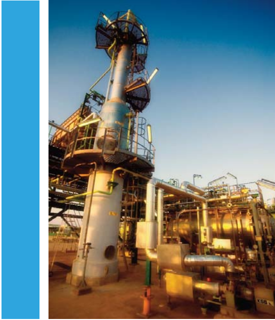
Planned expansion at the central processing facility at Temane forms part of the natural gas growth programme at Secunda
