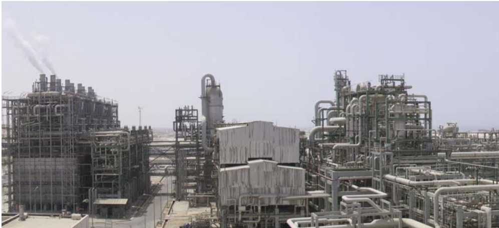
On 5 November the cracker portion of the Arya Sasol polymer project produced its first on-specification ethylene
