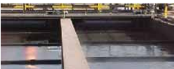
Rotary drum skimmers in operation at Natref
