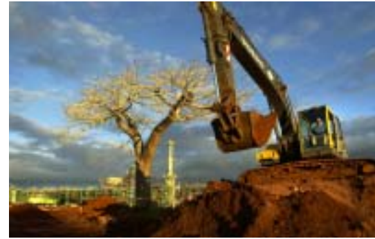
Central processing facility under construction in Mozambique as part of the natural gas venture.
