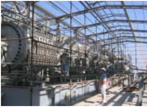
Arya Sasol ethylene cracker in Iran.
