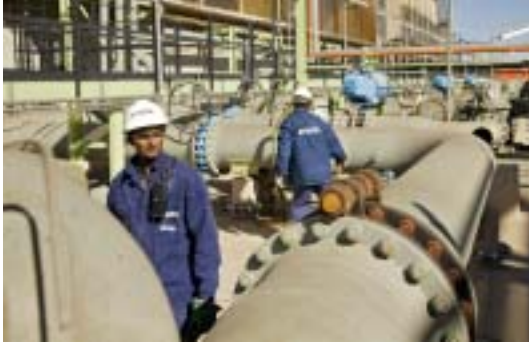
The Sasol Dia Acrylates facilities at Sasolburg.
