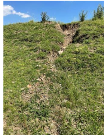
Erosion of overburden stockpile
