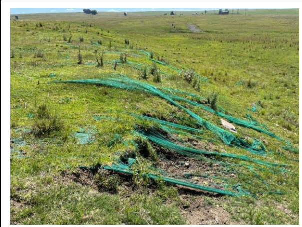
Erosion at the above stockpile area
