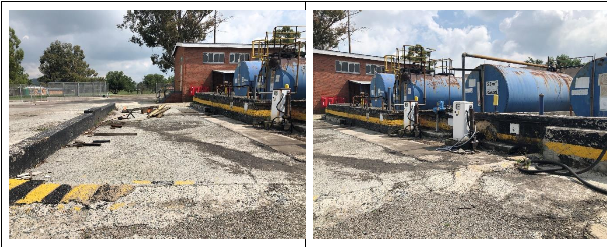
Bulk oil storage tanks
