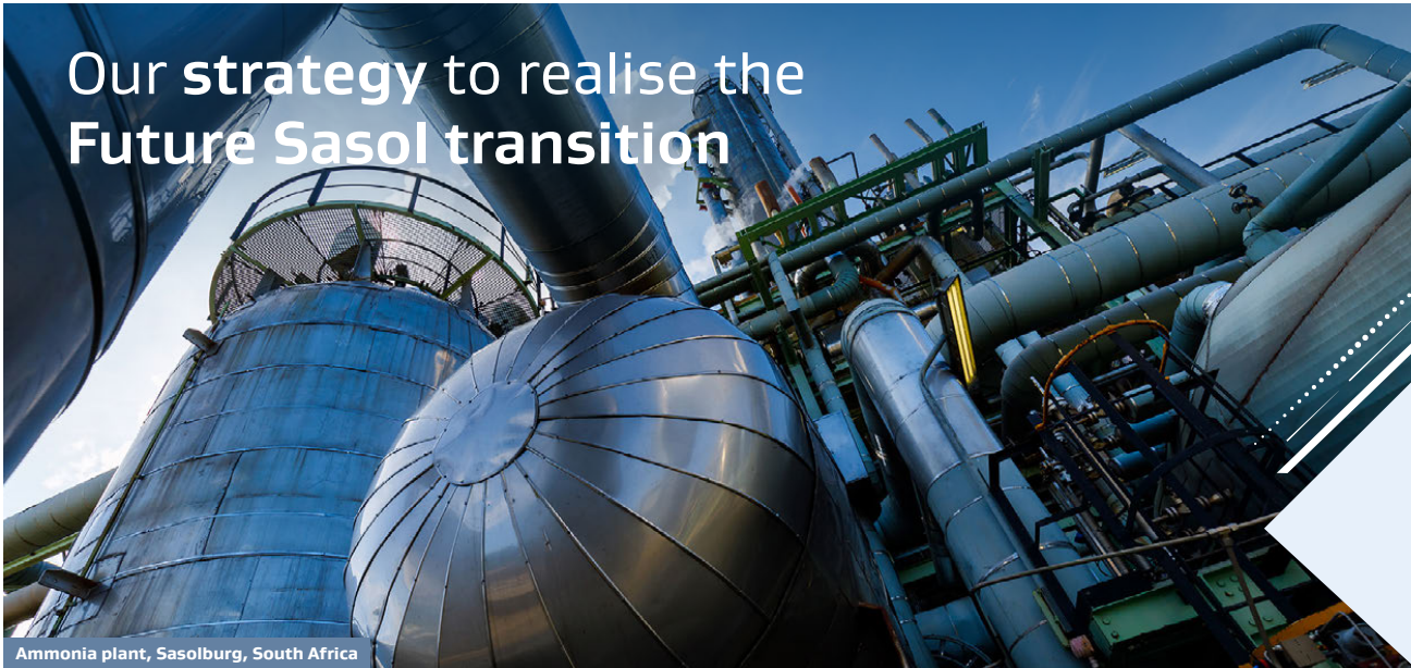
Ammonia plant, Sasolburg, South Africa
